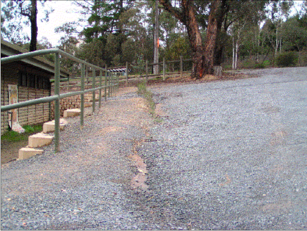
Appalling state of "car park" at rear of Deep Creek pavilion
