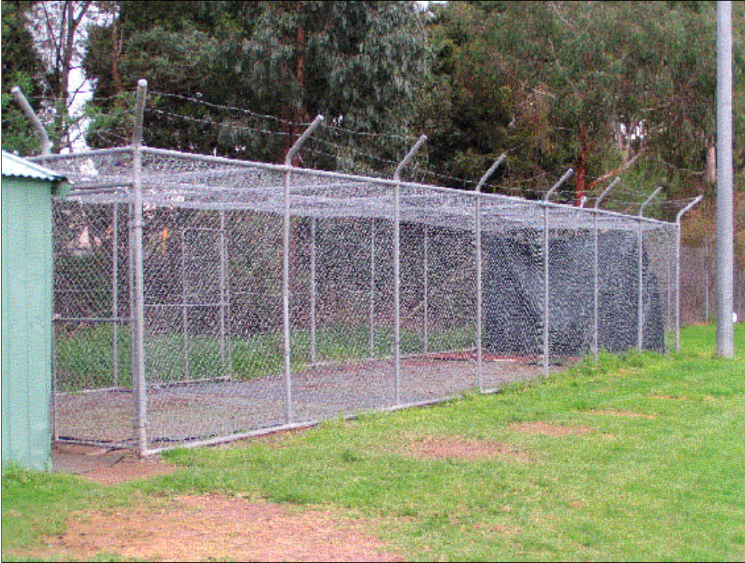
Dilapidated Batting Cage at Deep Creek Reserve
