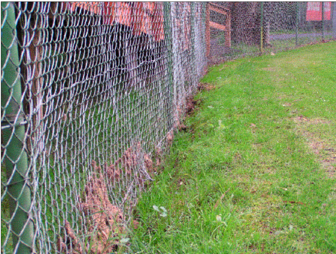
Dangerous “ditch” at foot of dilapidated Home Run Fence
