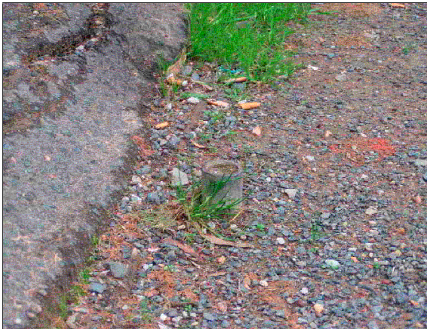
Sawn-off pole (one of four) protruding in front of pavilion
