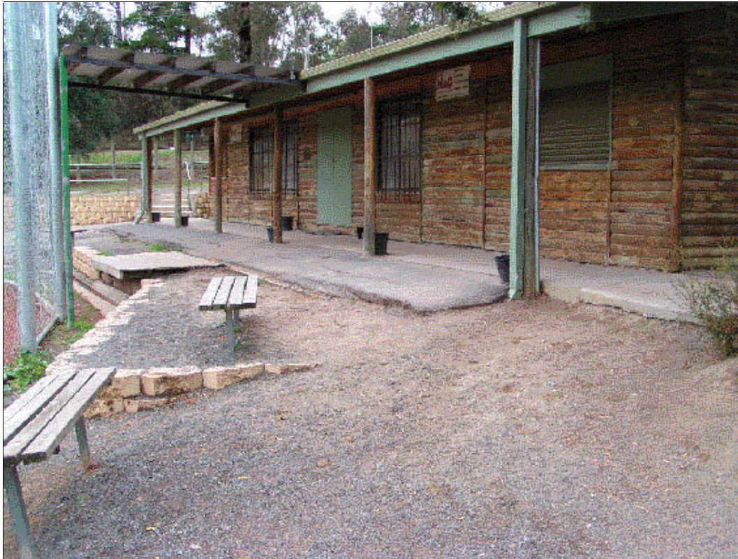
Poor state of front terracing (note the uneven, crumbling pavement, ageing timber deck and front door step restricting disabled access)
